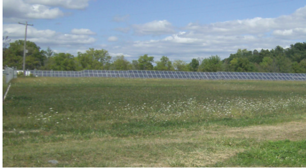
EXAMPLE OF GROUND MOUNTED SOLAR ARRAY IN FIELD
